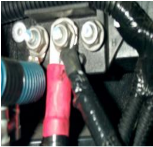
Incorrect Hookup Only 3 cables, can be on any of three lugs
